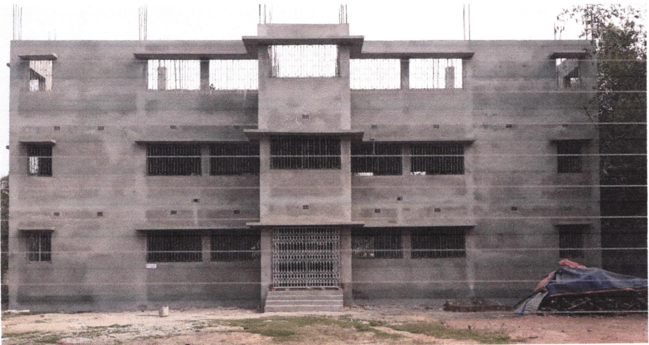
This above photo is showing the Current Construction stage as of 31 st March 2023
